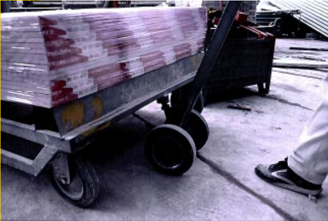
Purpose designed trolley for moving wallboard. Photo credit W A Browne Ltd
