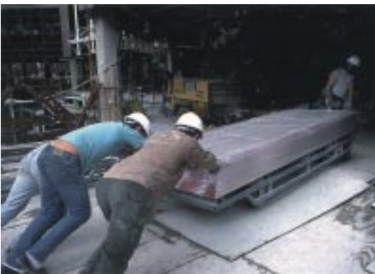
Purpose-made trolleys were used to convey gypsum wallboard in this development at Broadgate.
